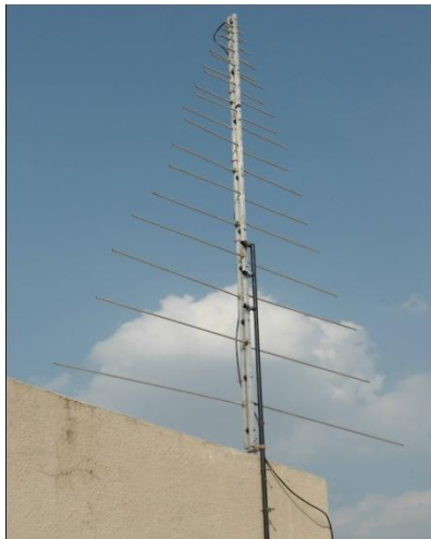
Fig2. LPDA installed on terrace of the building.
